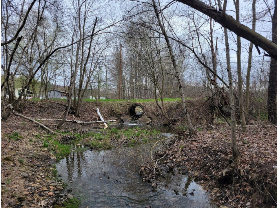
Figure 4: Photo taken of Whiteside Run just downstream of the culvert on Birch Road. There is a drop from the bottom of the culvert to the surface of the stream. This photo was taken in September. Whiteside Run was noted as dry when conducting culvert surveys in October.
