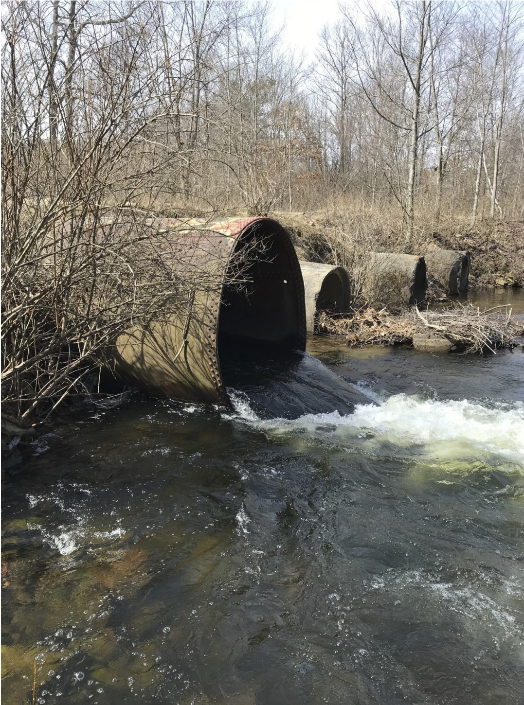
Figure 7. Outlet of crossing on Meyers Run Road on Black Moshannon Creek. Photo credit: Moshannon Creek Watershed Association.
