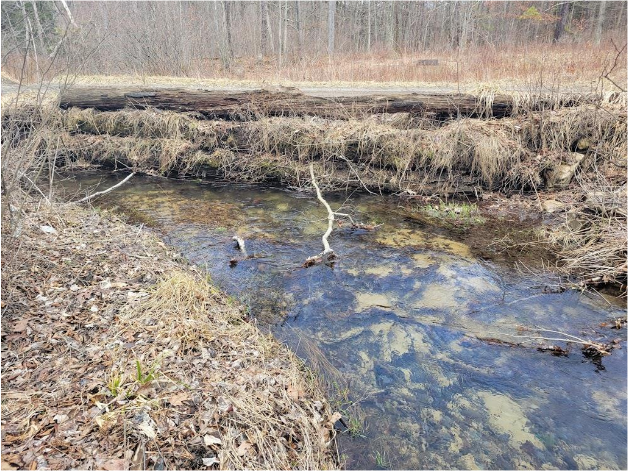
Figure 5b. Clogged and collapsed inlet of crossing with multiple pipes on Trim Root Run.
