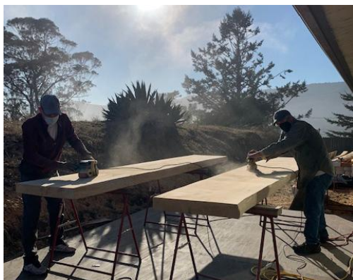
Keith and John seen sanding the wood planks. In the spirit of sustainable use of
