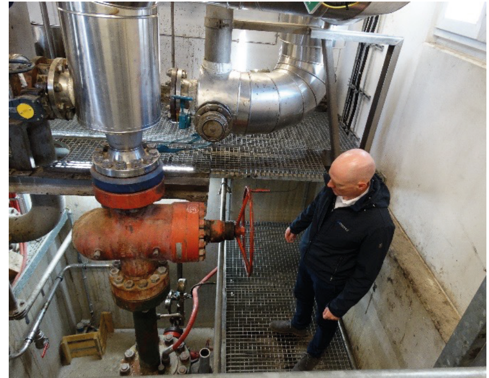
Viewing a deep geothermal well
