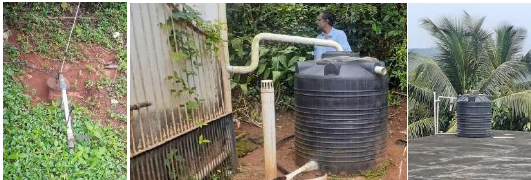
Bore well recharging point, Filtering Unit, and one Distribution tank
