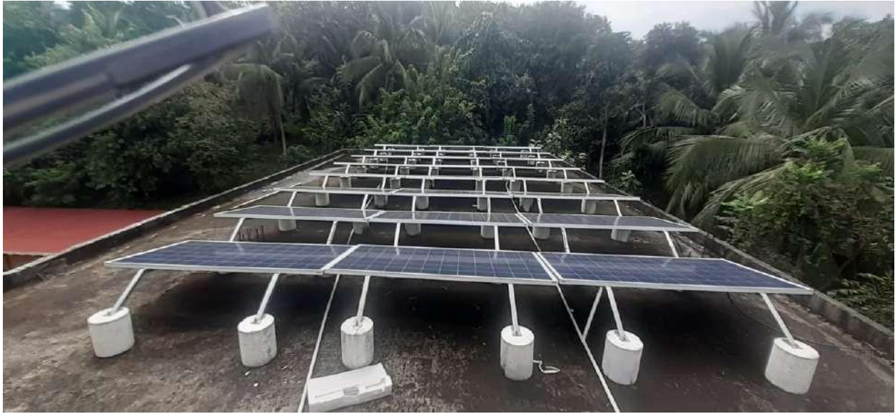
8.0 kW Solar PV plant at AMC Manisseri feeding the KSEBL grid
