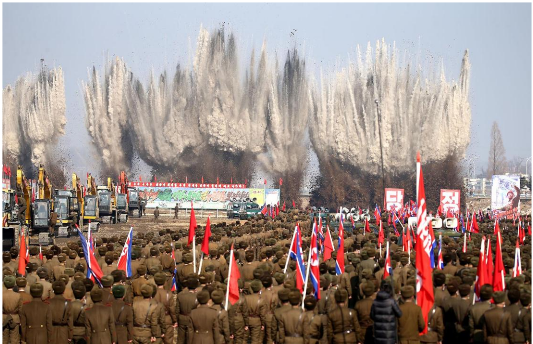
Groundbreaking ceremony held in February 2022 for building 10 000 flats in the Hwasong area
