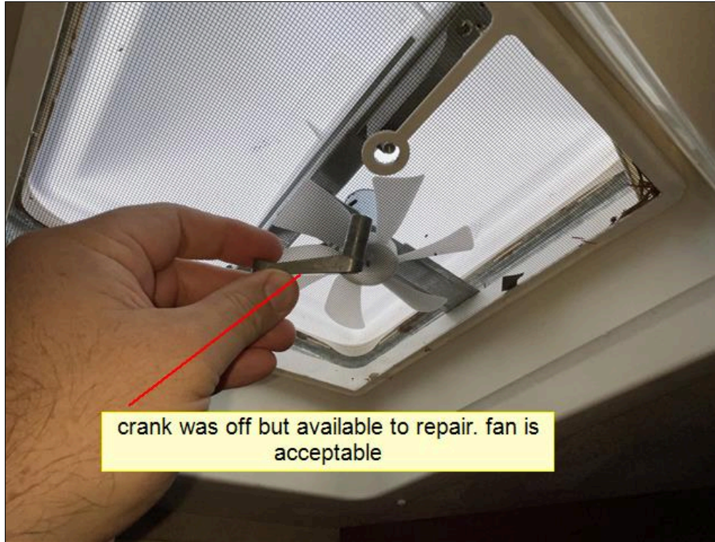
Bathroom manual crank vent
