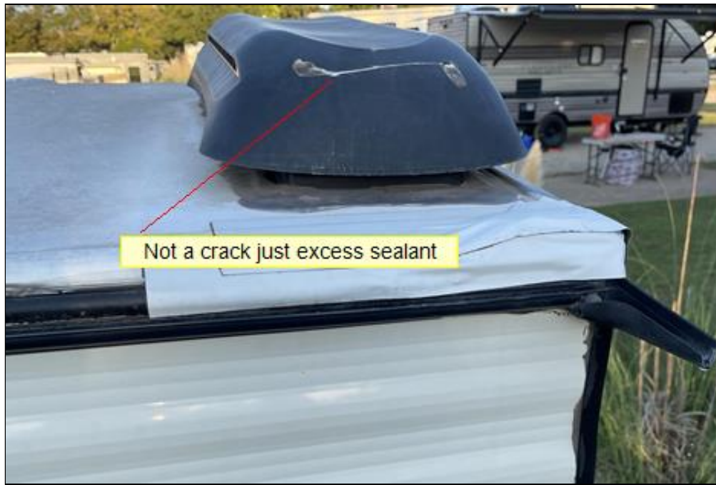
side view of roof refrigerator vent
