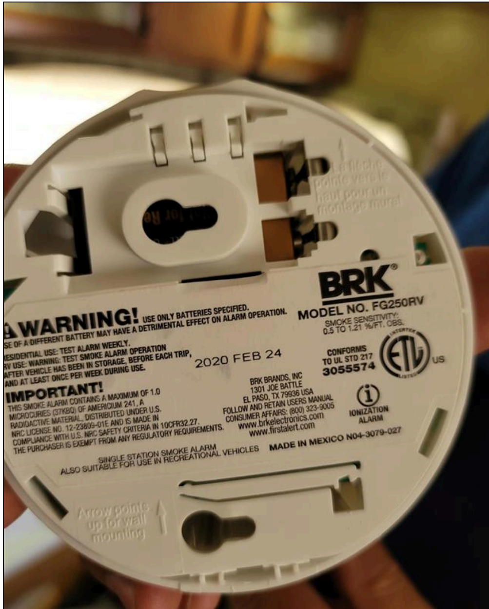
view of smoke detector
