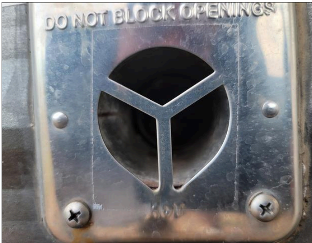
bottom furnace exhaust
