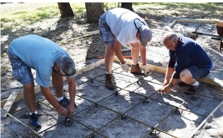
Manny Barros, Danny Elliott, and Pete Grasso prepare rebar for the cement.
