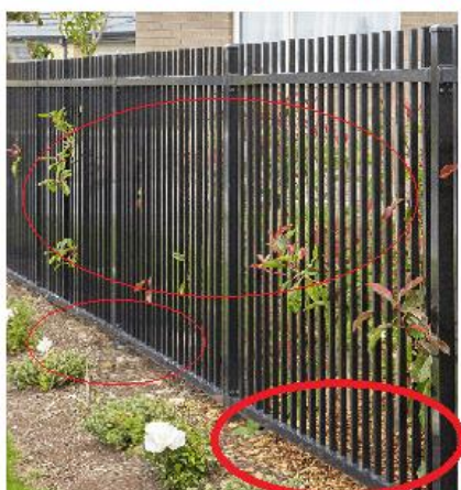
Not acceptable: Gap under and through fence
