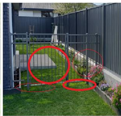
Not acceptable: gaps through the fence and underneath
