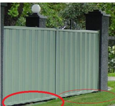
Not acceptable: Gap under fence requires a board
