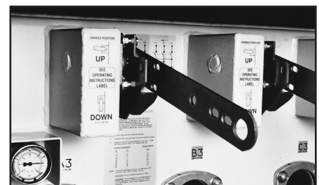
▲ Single phase interrupter operating handles.
