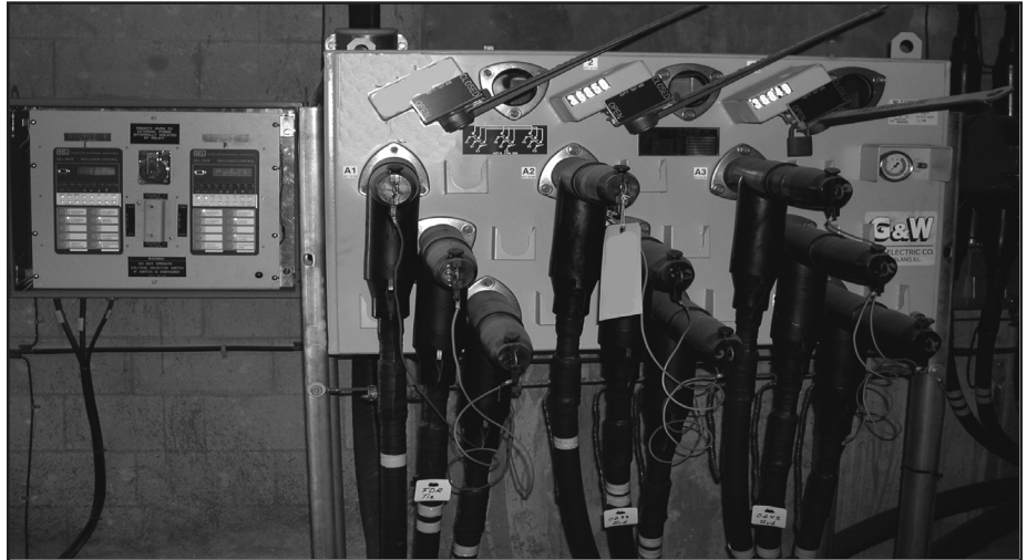
▲ Vault switch with SEL controls.
