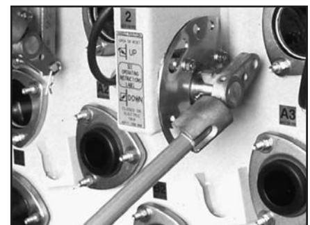
▲ Fault interrupter operating handle.
