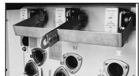
▲ Three phase interrupter operating handle.
