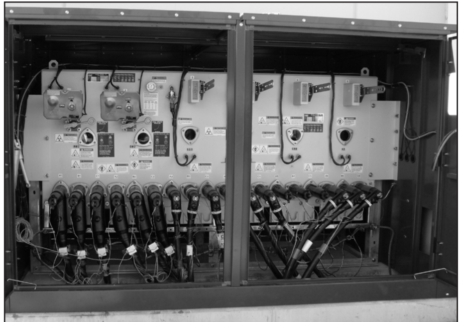
▲ Padmount switch with SEL controls.
