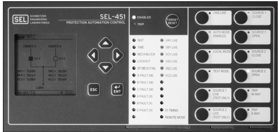
▲ ATC 451 control panel.
