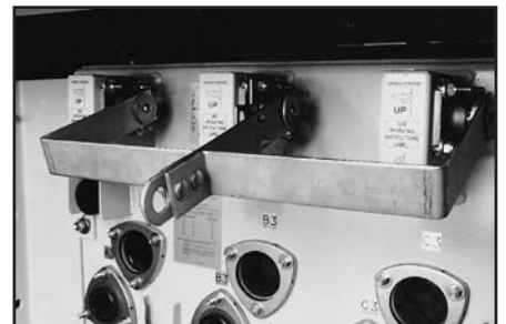
▲ Three phase interrupter operating handle.
