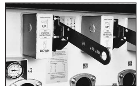
▲ Single phase interrupter operating handles.
