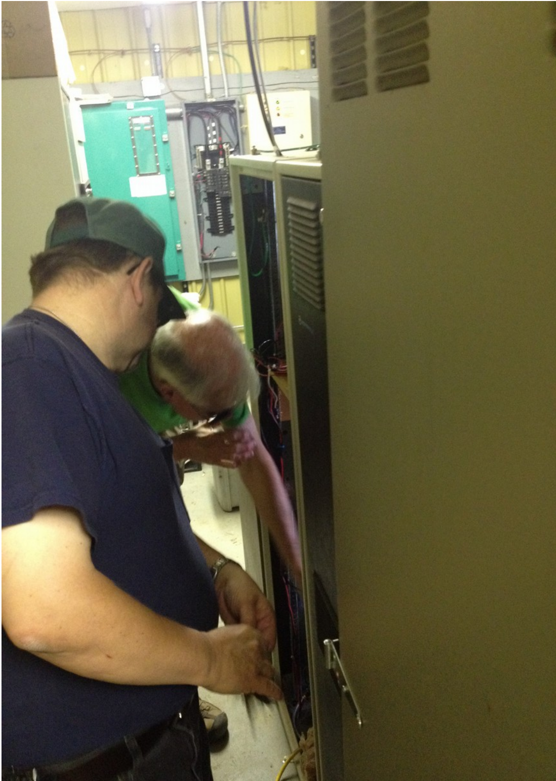
Ron (K2TJW) and Harold (N2FMS) working inside the cabinet
