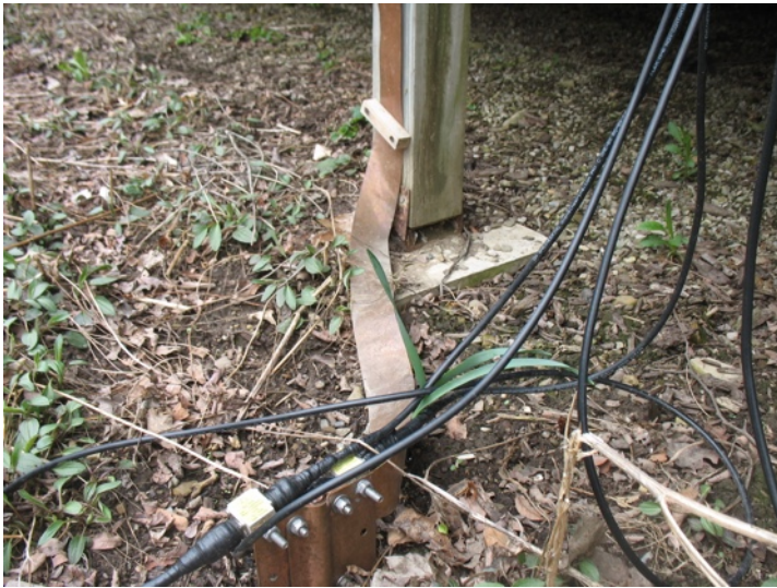
2" wide copper grounding strap bonded to a copper plate and ground rod. Attached to the plate are two lightning surge arrestors. One arrestor for each antenna coax feed line.
