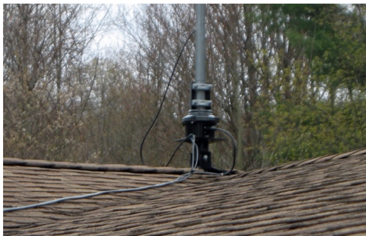
Roof mounted rotator turns the mast and antenna. No tower needed!
