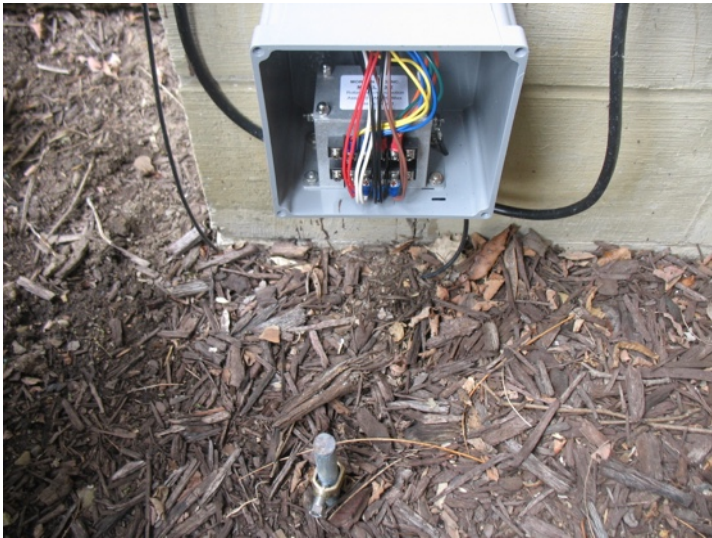
Rotator control line surge arrester mounted in a water proof box bonded to a ground rod.
