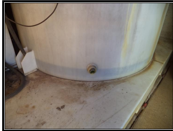
Photo No. 12: Bottom of one of the two larger tanks in air scrubber room, showing fluid level near the bottom.
