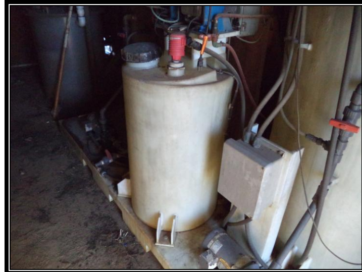
Photo No. 11: View of smaller tank in the air scrubber room.
