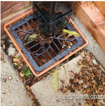
Item Muck In Round Downpipe Outlet
