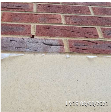
Item Some Plastic To Remove Above Rear Stone Work
