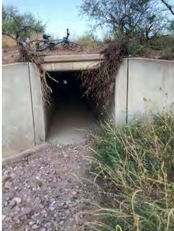
Box culvert under I-19 much larger than the 3 CMPs at Anza Trail ( outlet to river ). (Photo by Rich Kiker)
