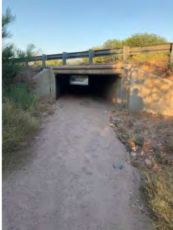
Box culvert at East Frontage Road also much larger than the 3 CMPs at Anza Trail ( outlet to river ). (Photo by Rich Kiker)
