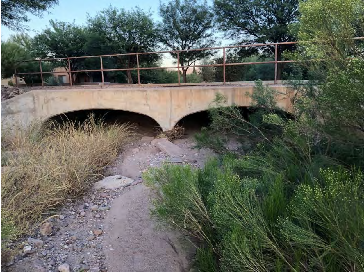
Arch culverts under Paseo de Tumacacori. Possible sediment build-up likely reducing hydraulic capacity.
