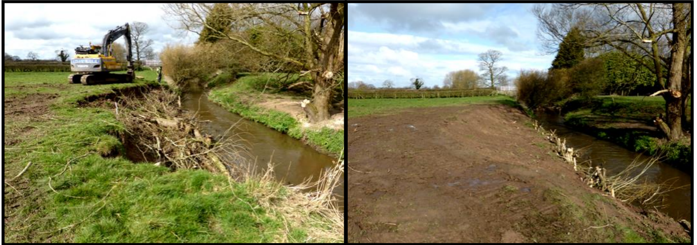
Left - Willow branches and brash tethered to bank - Right - Erosion scar backfilled and graded.
