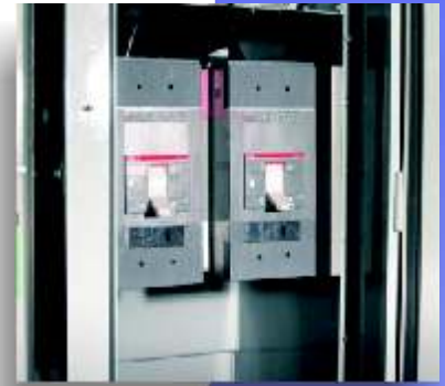
Low Voltage Breakers
