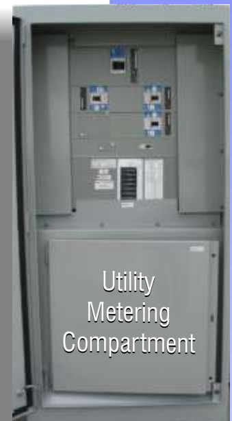
Side Distribution Panel with Utility Metering Compartment
