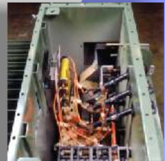
Bay-O-Net and backup current limiting fusing
