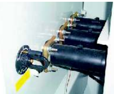
Air/Water Tight Switch Connection
