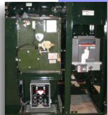
MiniSub with Primary Auto Transfer Switch
