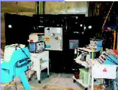
Final Testing Bay
