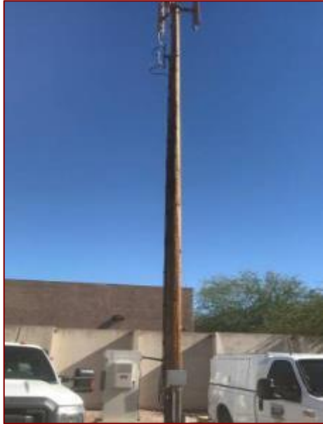
Head End Node Placed Next to Pole with Antennas
