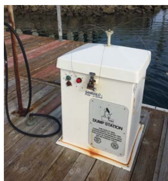
Dump station installed remotely from point of service Photo by TBF
