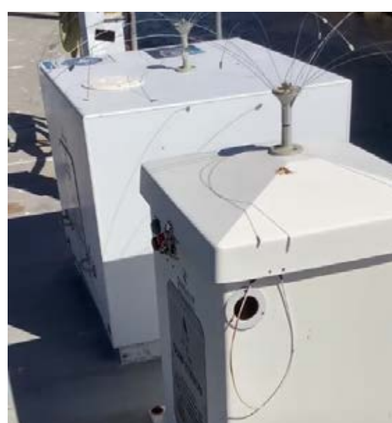
Dump station (right) installed at the point of service Photo by TBF
