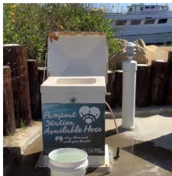
Gravity-drained dump station in Santa Barbara Harbor Photo by TBF
