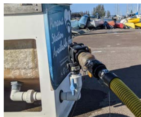
A gravity-drained dump station manually connected to a pumpout unit’s infrastructure by attaching the pumpout unit’s hose to the dump station waste fitting Photo by SFEP
