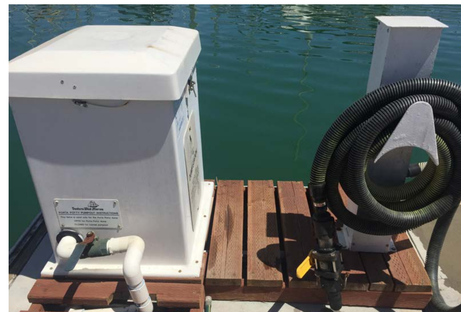
Motorized dump station requiring the manual opening of its ball valve for drainage Photo by TBF
