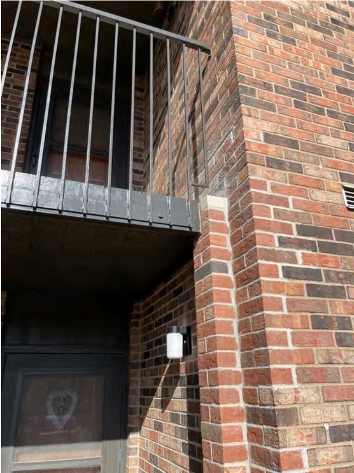
5. Additional masonry cleaning required above new pier at Building A1.
