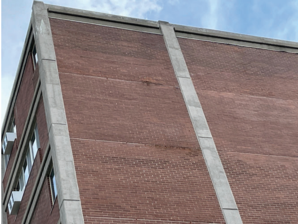
3. Multiple panels hosting bulging brick.
