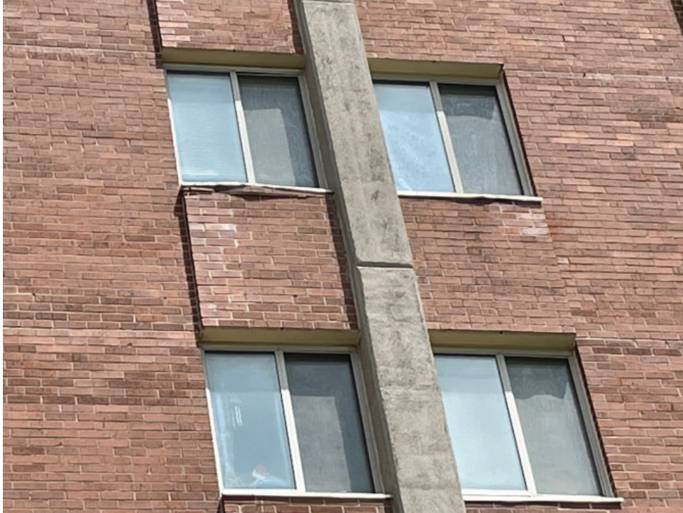
5. Pinched brick and damaged sill at south-facing window at Building A.
