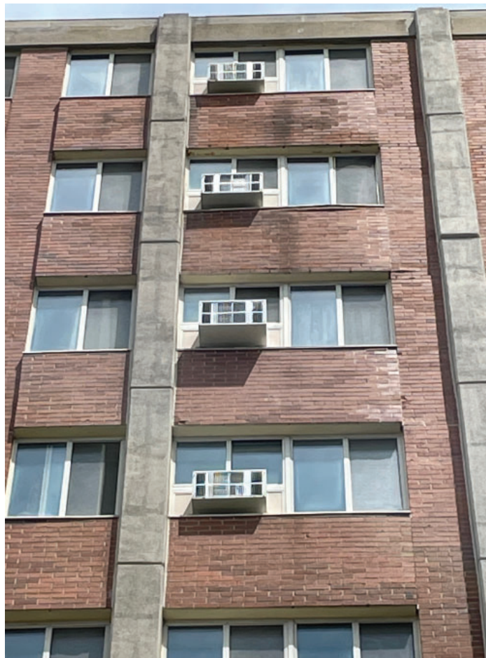
6. Pinched brick below window.
