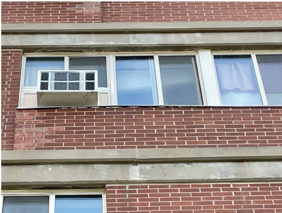
4. Damaged sill and masonry below.
