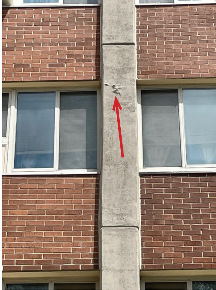
7. Peeling of concrete column coating.
