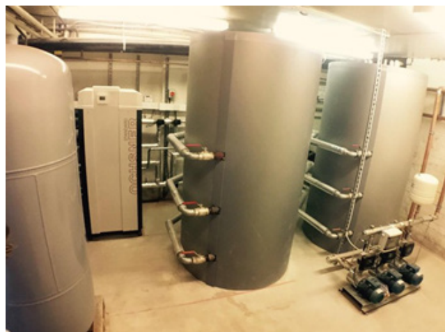
Example Communal ASHP Internal Plant Room
