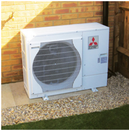
ASHP Mounted Externally
