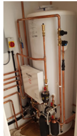
HWS Cylinder and Associated ASHP System components within cupboard inside dwelling
