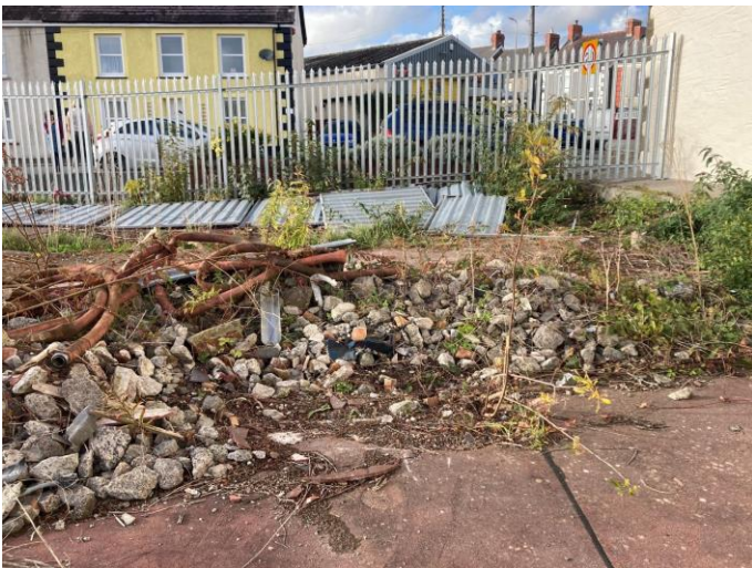
9. Debris piles in NW corner
