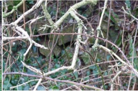
Stone wall with gaps in stonework – located along southern and western boundaries
