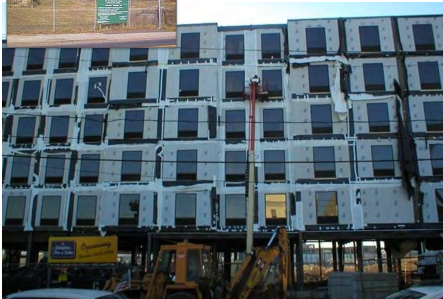
Before (above left) and during redevelopment of a hotel in Hudson County, New Jersey.
