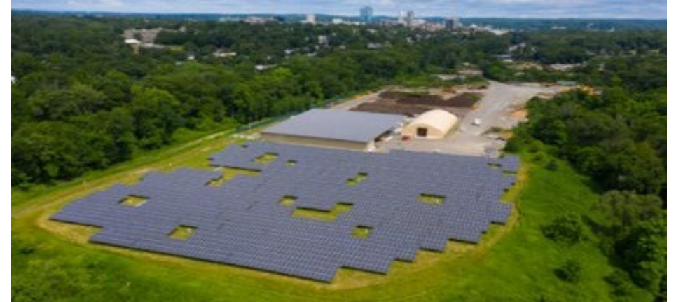
Floating foundation canopy mounted on a landfill cap at the Gedney Way Recycling Facility
