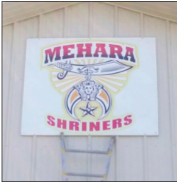
On Member's Workday, a new club sign was installed on the peak of the Mehara Shrine Club building.
