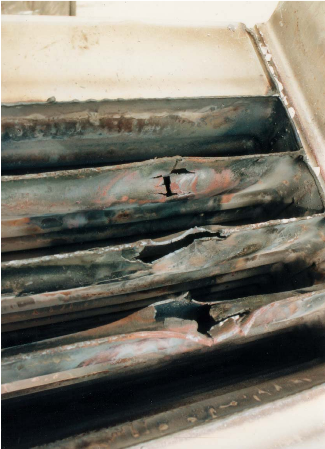
Photo Six: Failed heat exchanger.
