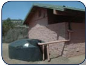
Acker Park System installed 2007
