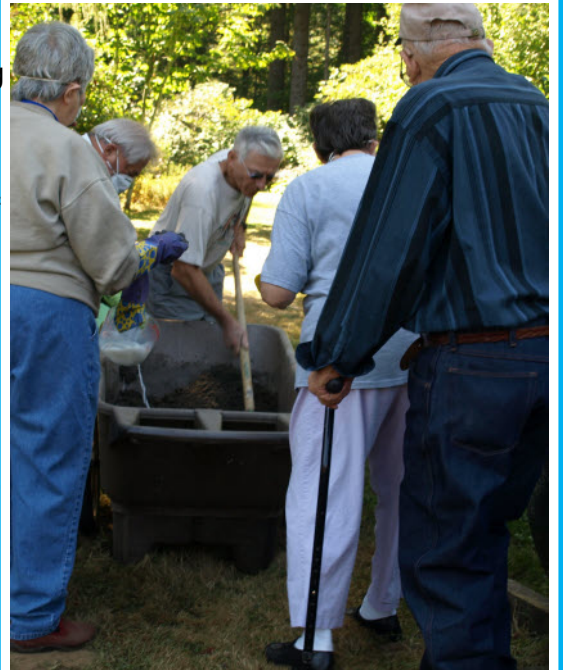
JoAnne, Helen and Galen Baxter watch A. J. Giustina pour in the admixture as Jack Olson stirs the thick mixture.
