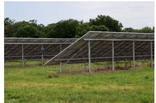
Example of a Solar Conversion System, Ground-mounted
