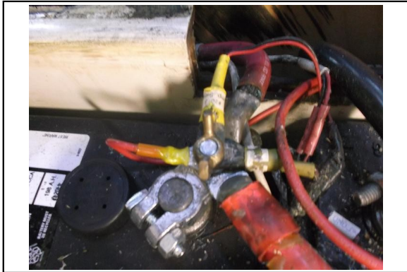
No Overcurrent Protection
