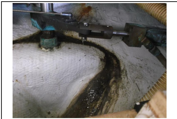
Leaking Rudder Post
