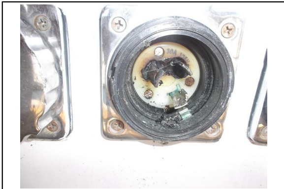
Shore Power Inlet 1
