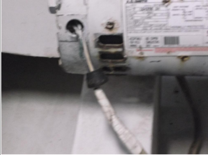
A/C Pump Wiring
