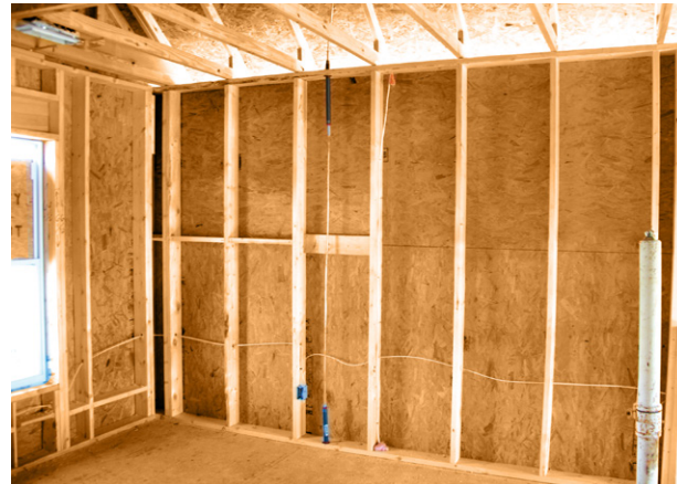
2x horizontal blocking between studs can be oriented with either the edge against the sheathing/drywall or the wide face vertical against the sheathing/drywall. Both options are shown.
