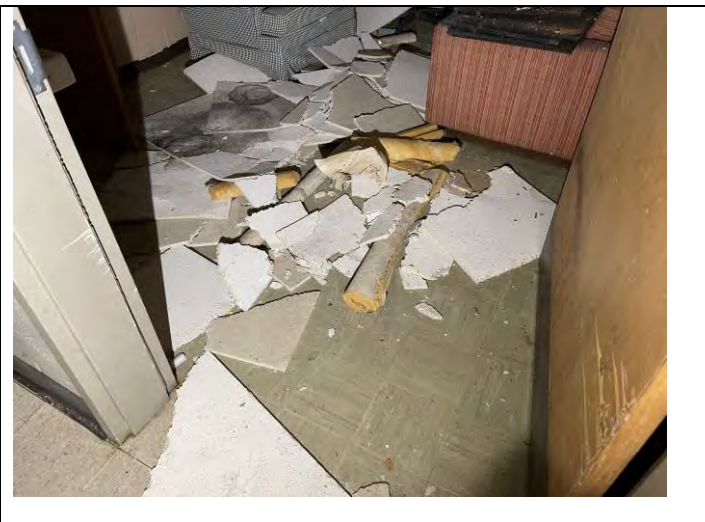
17. Pipe Fitting Insulation (Intact and debris on floor)
