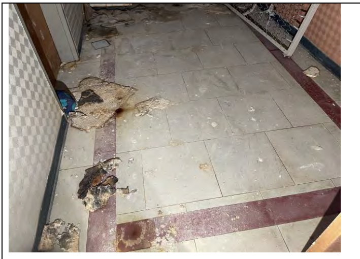
9. Black Mastic under Various Sizes of Floor Tile
