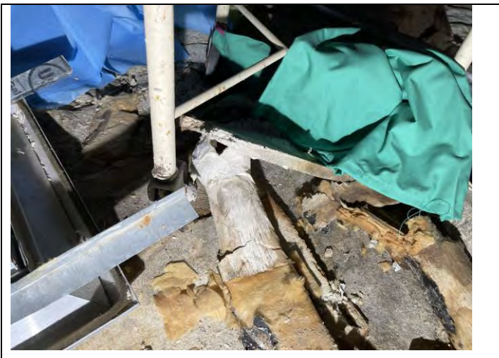
29. Pipe Fitting Insulation (Intact and debris on floor)
