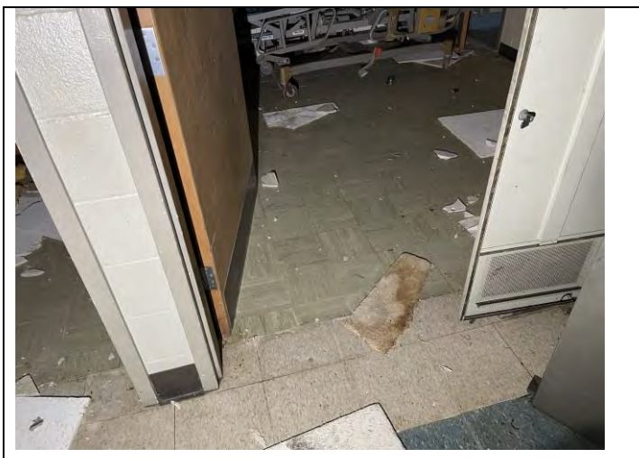
5. Black Mastic under Various Sizes of Floor Tile
