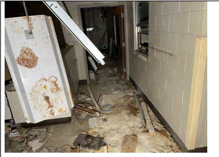
27. Pipe Fitting Insulation (Intact and debris on floor)
