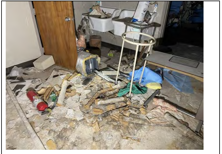
28. Pipe Fitting Insulation (Intact and debris on floor)
