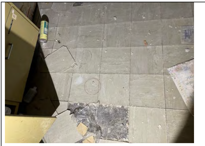
3. Black Mastic under Various Sizes of Floor Tile
