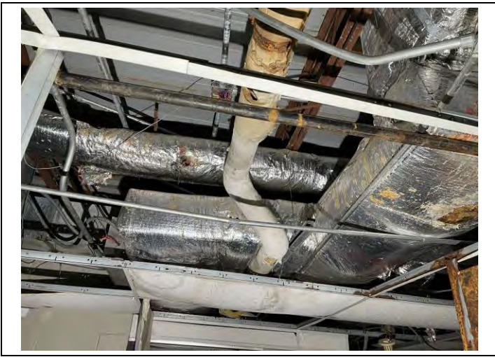
25. Pipe Fitting Insulation (Intact and debris on floor)
