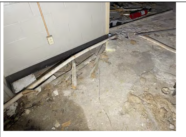
23. Pipe Fitting Insulation (Intact and debris on floor)
