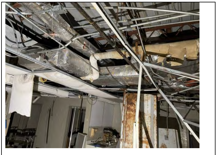
24. Pipe Fitting Insulation (Intact and debris on floor)
