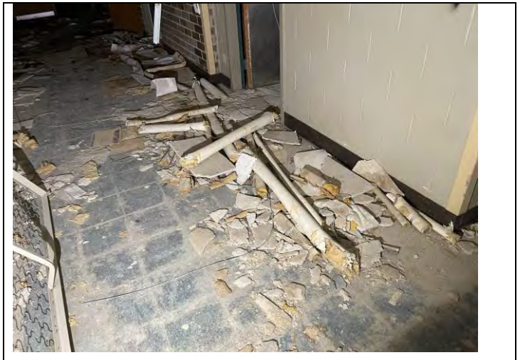
22. Pipe Fitting Insulation (Intact and debris on floor)
