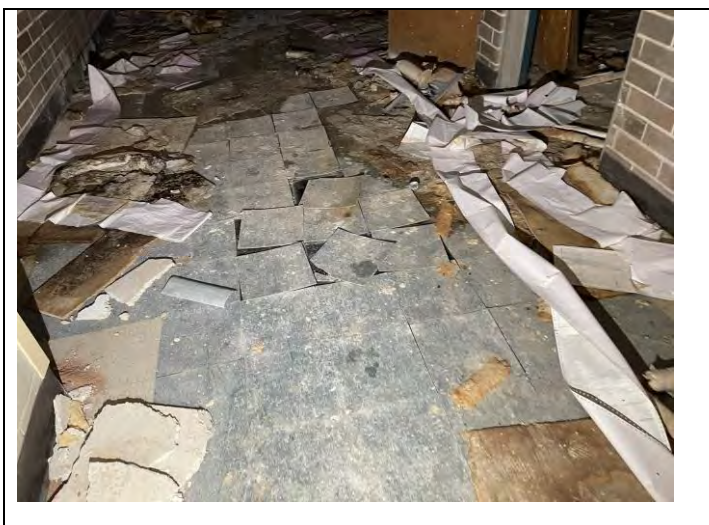
11. Black Mastic under Various Sizes of Floor Tile
