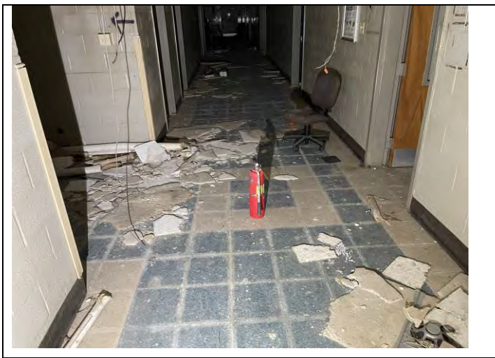
7. Black Mastic under Various Sizes of Floor Tile
