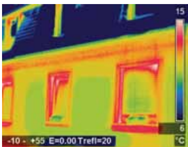
The warmest areas seen here in red show where heat is being lost from the building.
