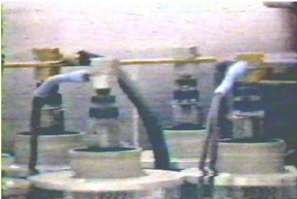
Ignitrons installed on the "Red Motor Cart"
