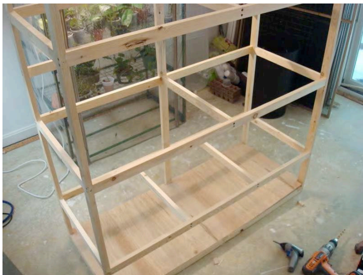
Figure 1: Here is the frame with shelf supports assembled. The very bottom is a tiny shelf made of 1/4" luan plywood that will be outside of the watertight enclosure.
