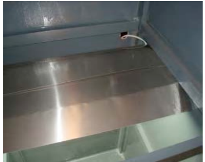
Figure 6: Aluminum flashing above light prevents dripping water from contacting fixture. Note hole in upper left corner for cord exit.
