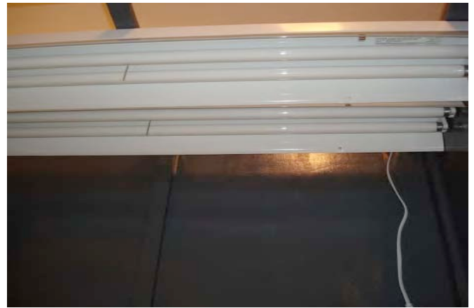
Figure 5: Lighting installed on bottom of shelves and top of chamber.
