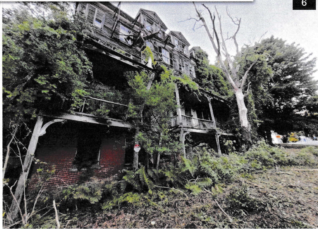
Photos 5 and 6: (5) Showing the porch/ deck structures along the West Road side of the building, state of disrepair and unsafe conditions. (6) Example of the vegetation which had previously been on the structure and contributing to the decay.
