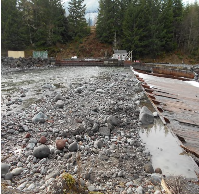
Bedload stacked upstream of Diversion structure
