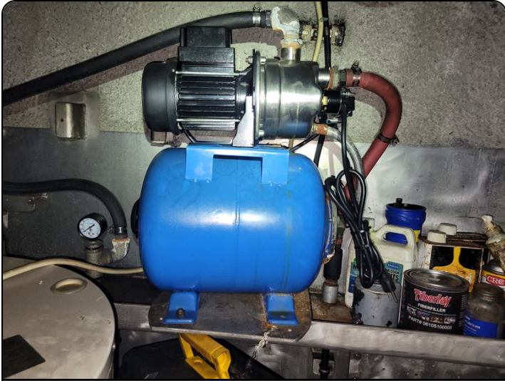
Photo 29: 110 VAC Freshwater System
