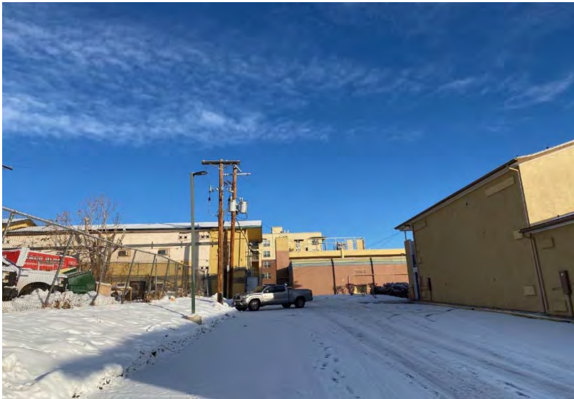
View of pole-mounted transformers along the southwest border of the subject property. View to the north.
