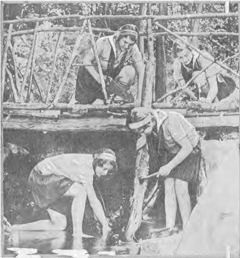
Campfire Girls repairing the damage caused by beavers to the rustic bridge made by them across the brook at their camp in Harriman State park, New York. Industrious beavers ate away the living trees which formed the natural supports at the land ends of the bridge.
