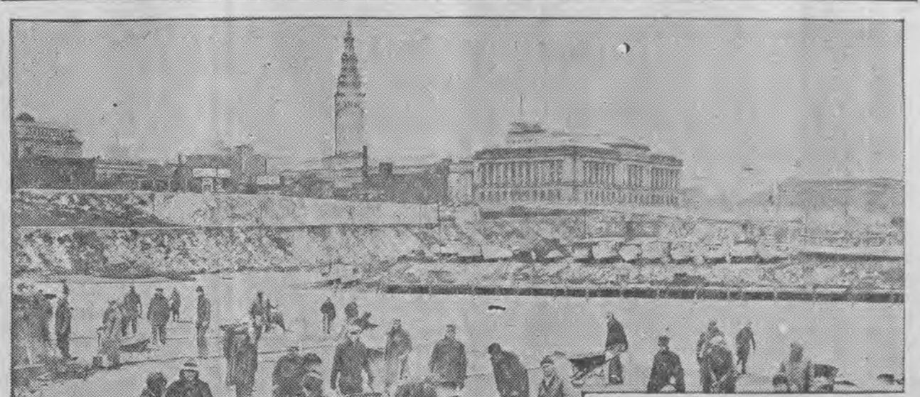
HERE are some of the hundreds of CWA workers who are employed in building a lakefront airport for Cleveland, Ohio. It will be one of the few in the country situated within a mile of a city's business section. The project, sponsored by City Welfare Director David S. Ingalls, calls for the expenditure of $250,000.
