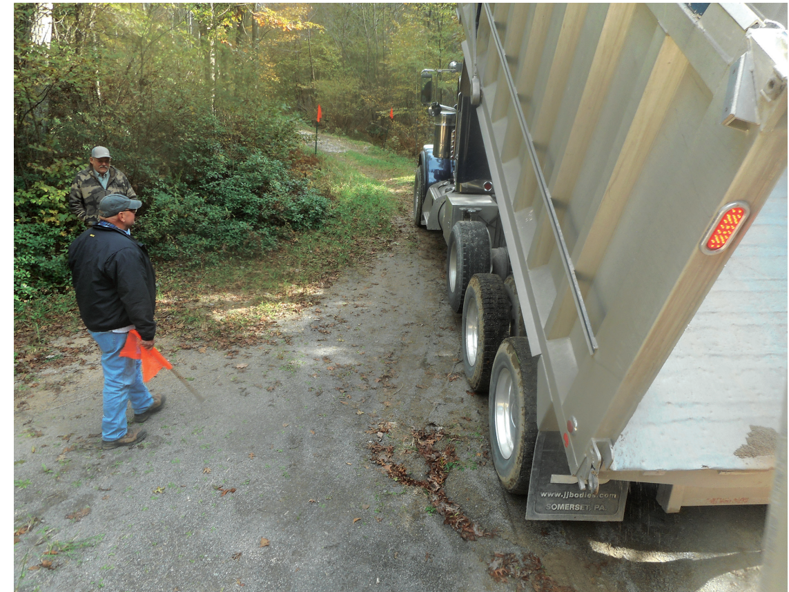
CRTU members John Gulya (with flag) and Al Crawford direct a 22-ton load of limestone sand through a "tight spot" to the acid remediation site on Glade Run main stem.
