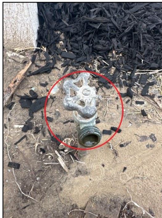
56. Backflow prevention missing
