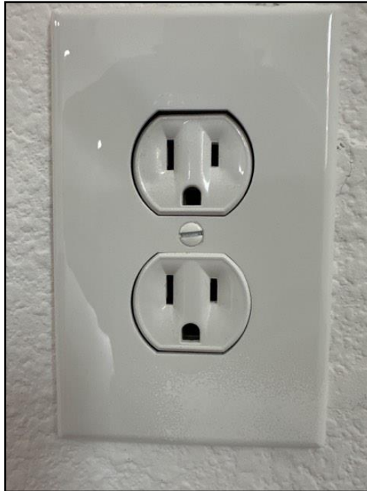
38. Receptacle within 5 ½ feet of floor not...
