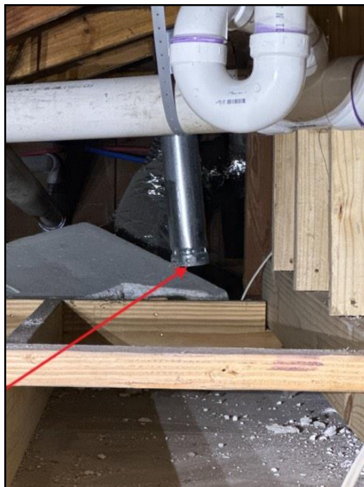
68. Not vented to exterior
