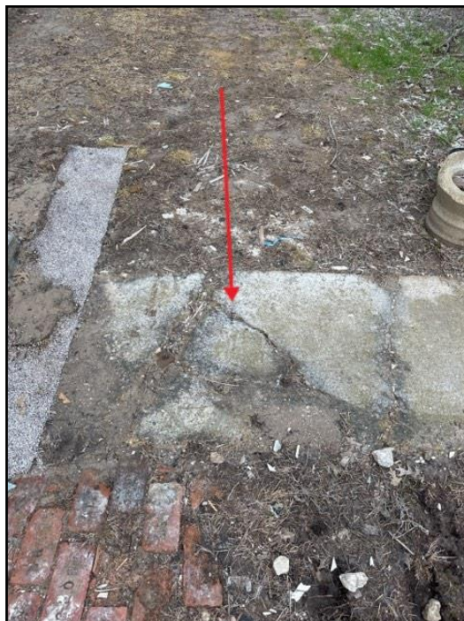
20. Cracked or damaged surfaces
