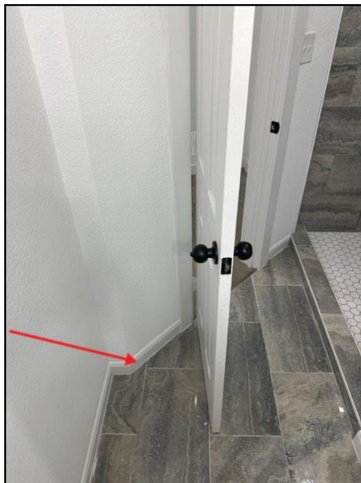
66. Doorstops missing or ineffective
