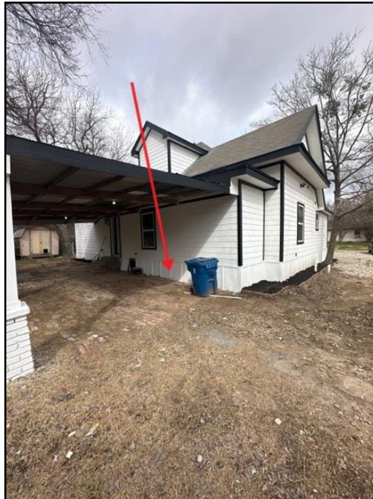
19. Improper slope or drainage
