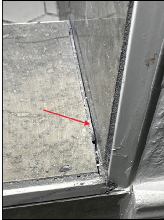
57. Grout loose, missing or deteriorated
