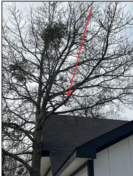
3. Tree branches touching roof
