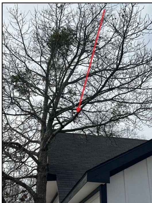
12. Tree branches touching roof
