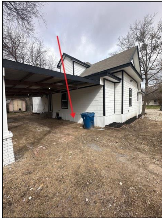
28. Improper slope or drainage
