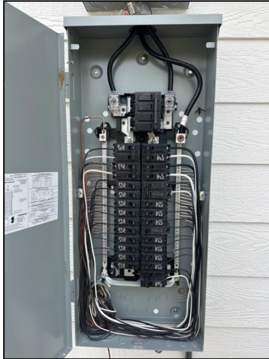
38. Breakers - exterior wall
