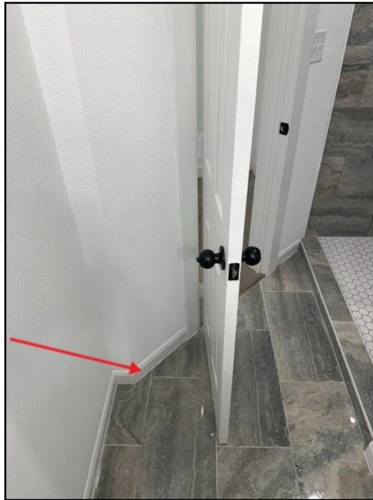
88. Doorstops missing or ineffective
