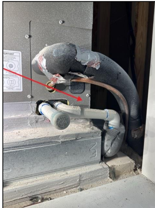
66. No float switch
