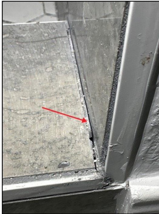
79. Grout loose, missing or deteriorated
