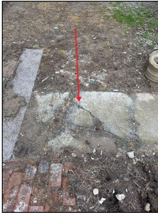
29. Cracked or damaged surfaces
