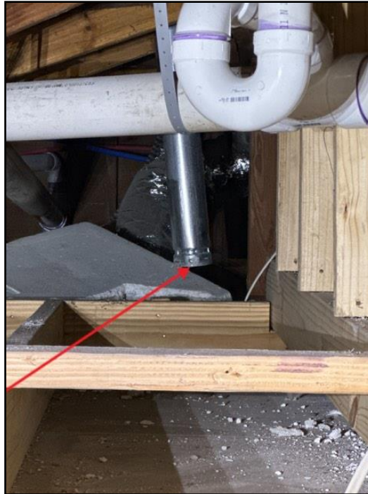
90. Not vented to exterior
