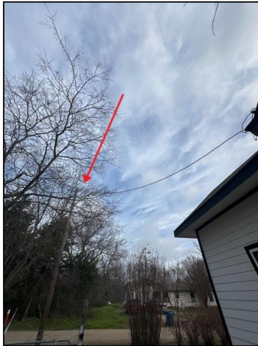
40. Branches / vines interfering with wires
