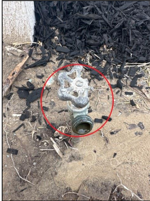
78. Backflow prevention missing
