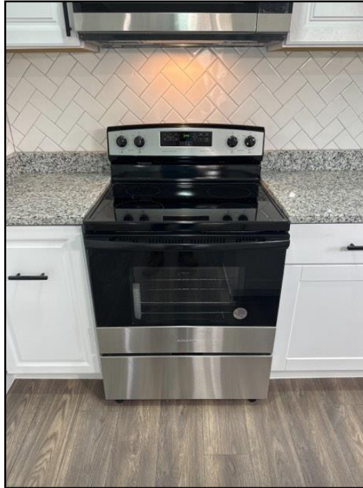
91. Anti-tipping device missing
