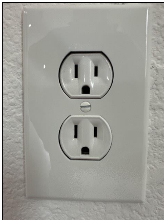
51. Receptacle within 5 ½ feet of floor not...
