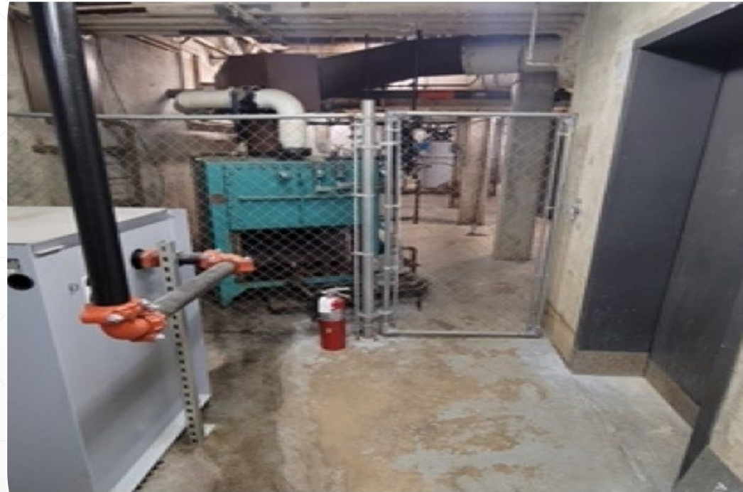
Fence Guard at Elevator
