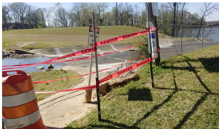
Spillway and sinkhole, looking west
